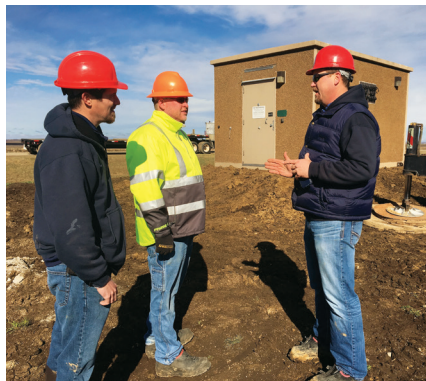
Alliance technicians Tom Chase, Dave Wirkus and Andy Hulscher discuss plans for installing a building for housing electronic equipment.
