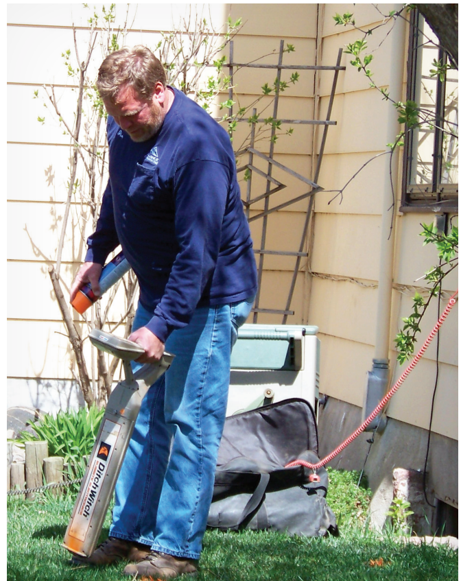
Jim marks underground lines at a home prior to burying new fiber-optic lines.
